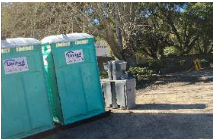
Two unsightly Job Johnnies inhabit this Lost Valley substation.
